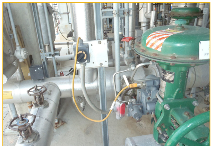
Figure 4. The site’s code expert insisted that power was removed from a device before uncoupling the “minfast” quick connect. But the internals of these disconnects sometimes became corrupted by the weather. A hermetically-sealed disconnect switch removes the power so a quick connect can be removed without a hot work permit.
