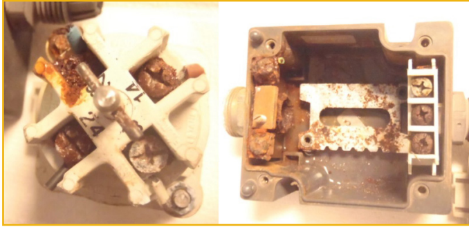
Figure 5. Corroded terminals became a concern and were suspected of causing communication issues.
