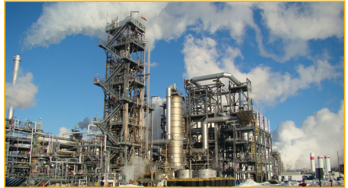
Figure 1. Ashland's 1,4-butanediol plant in Lima, Ohio has an annual capacity of 65,000 metric tons of BDO.
