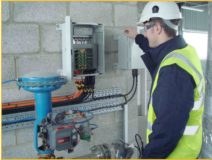
Figure 3. Fieldbus end users must be mindful of physical layer requirements such as power conditioning and segment termination.
